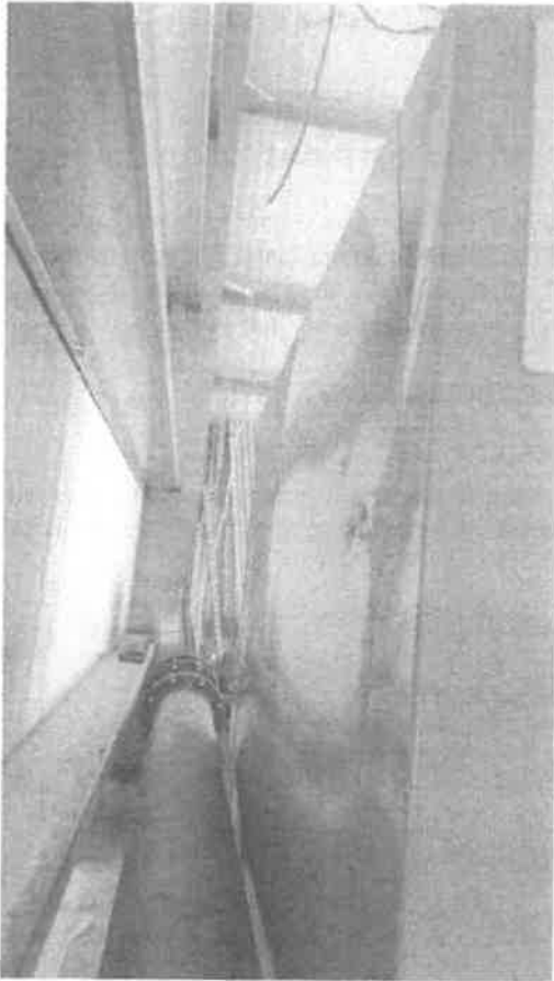
Figure 2 – Rear of GAC Pump Control Panel
